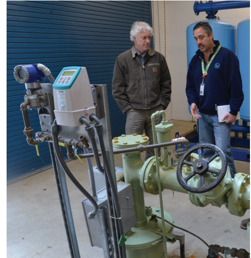
Sammamish Plateau Water Superintendent, John Anderson (right), explains why air/vacuum release valves need screening material on discharge piping during a recent visit with Derek Pell from our Northwest Regional Office.
