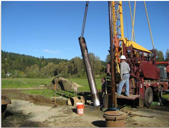
The well drilling contractor working on installing the production well as part of Phase 1 construction funded by the Department of Ecology.
