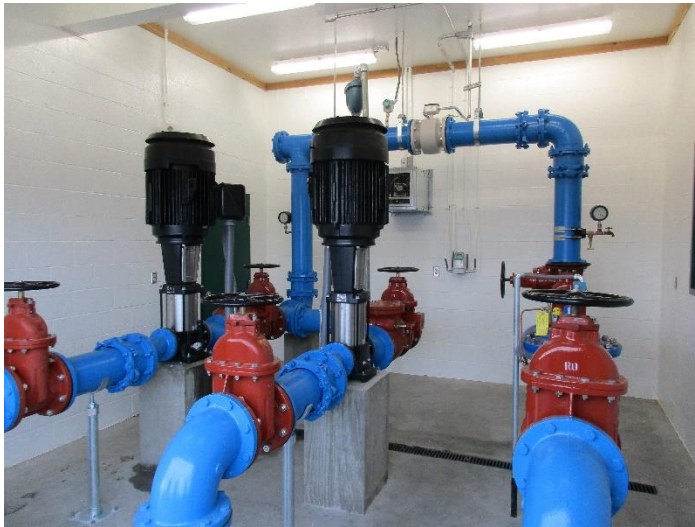
New booster pumps
